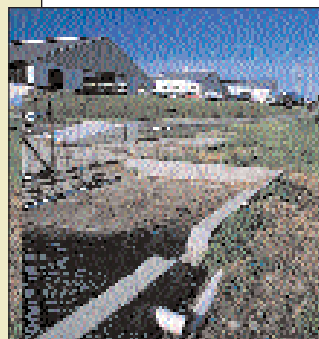
A curb and overflow pipe, such as this one at Table Rock Farm, Castile, N.Y., helps prevent bunker silo runoff from being an environmental hazard.
